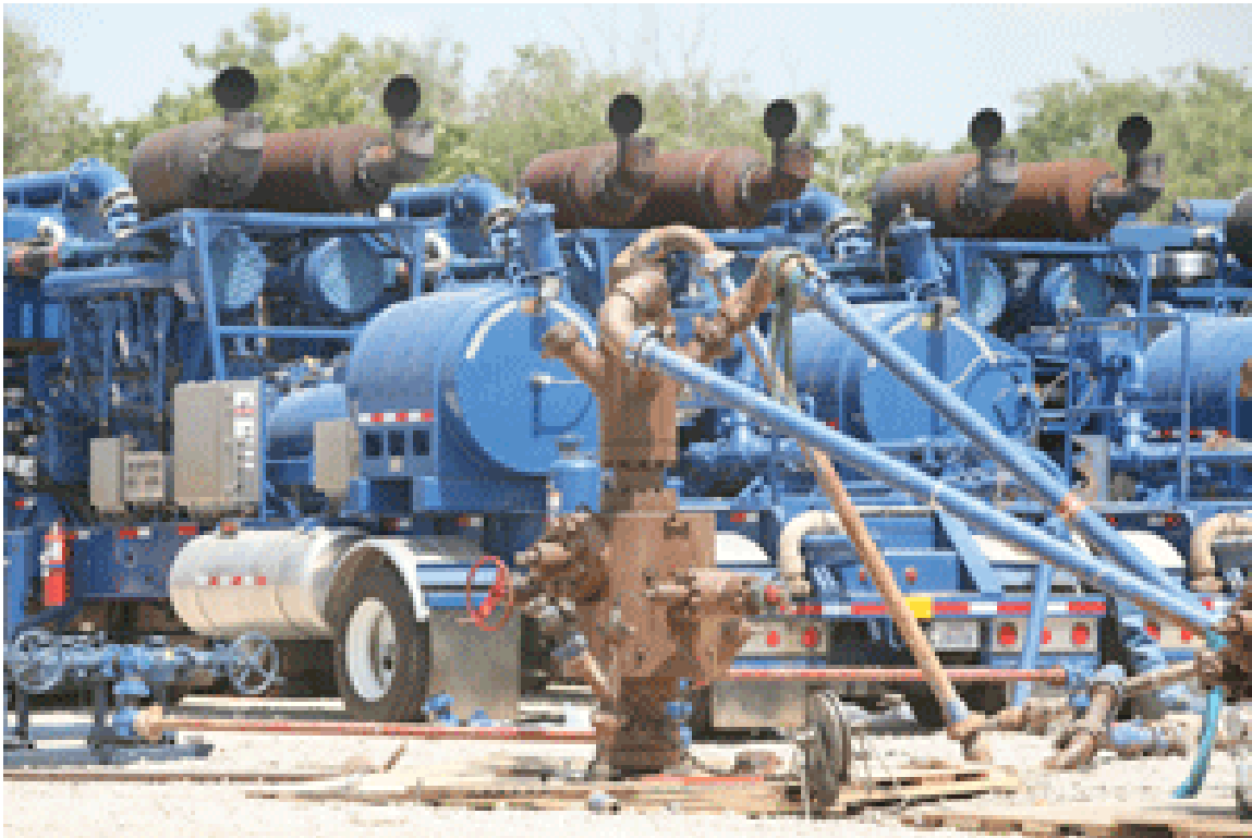
Compressors and heavy equipment can run 24/7
