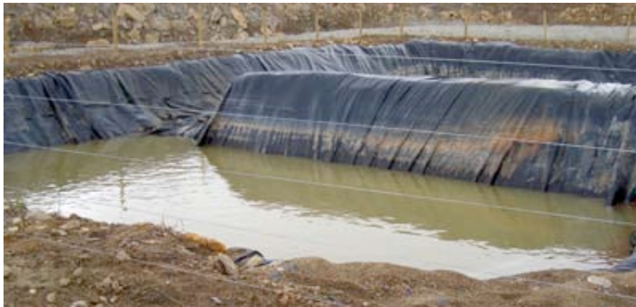
Open lined pit prone to seepage, ruptures and overflowing during heavy rains.
